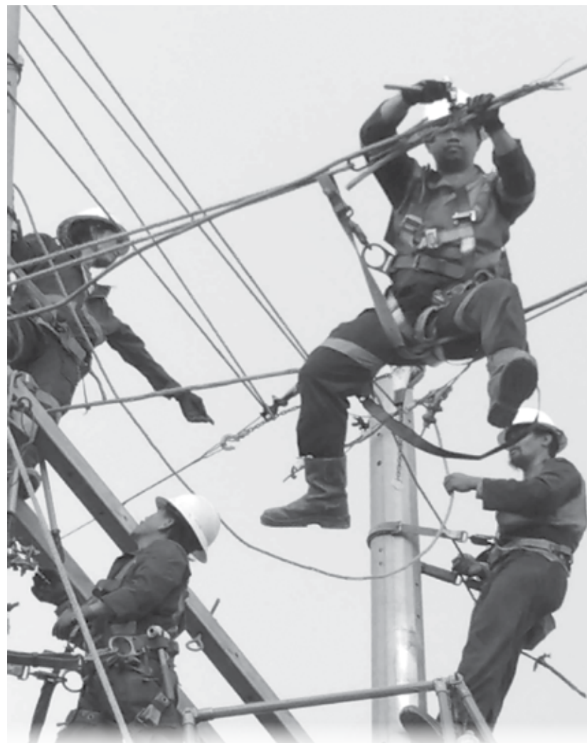
ALL DAY, ALL IN. The electric cooperative's linemen fix the lines to ensure the continuous supply of electricity to all households and businesses.
